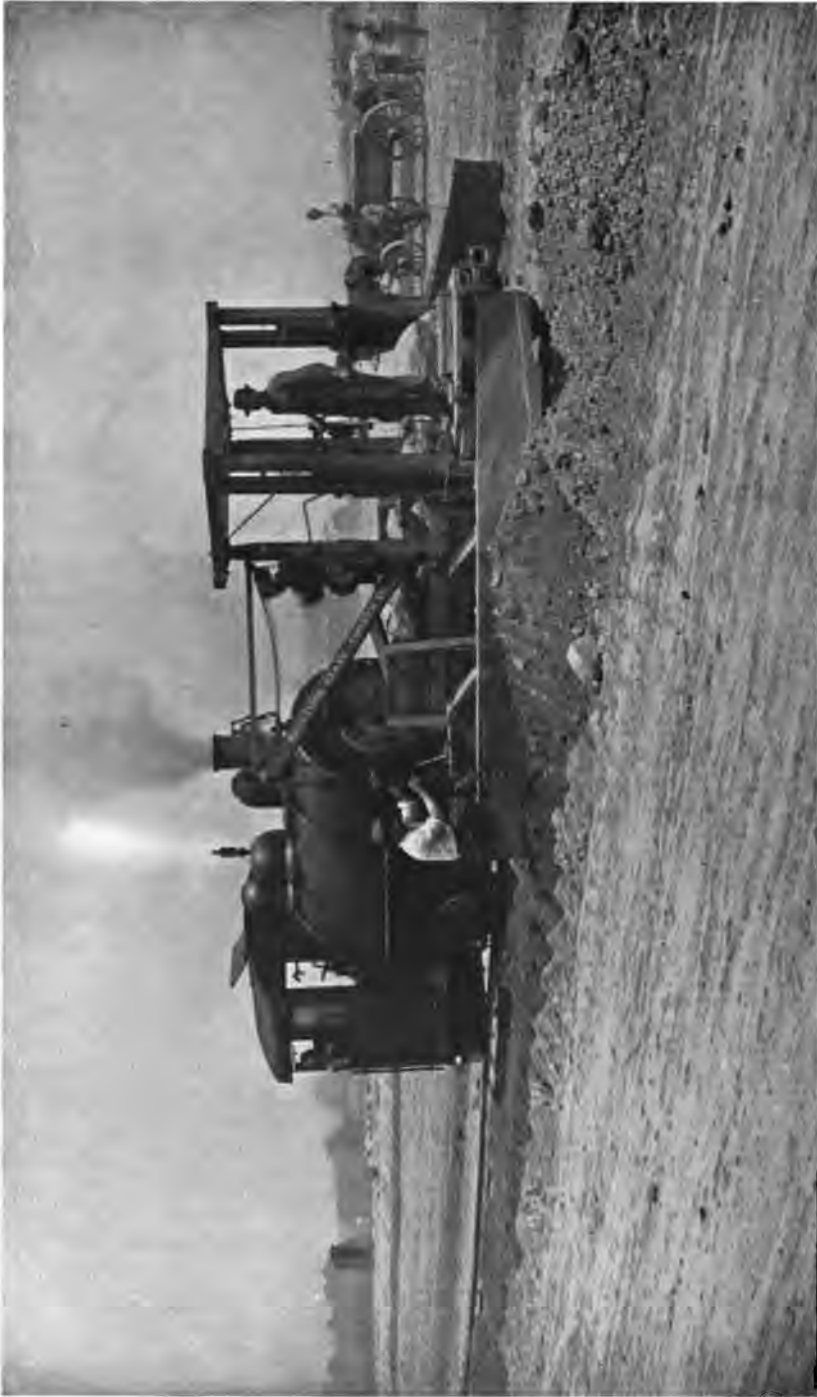
PLATE 196. —Hill View Reservoir. Spreader Used for Reducing Material Dumped from Cars to Proper Thickness for Rolling by Steam Roller to Make Impervious Embankment.
